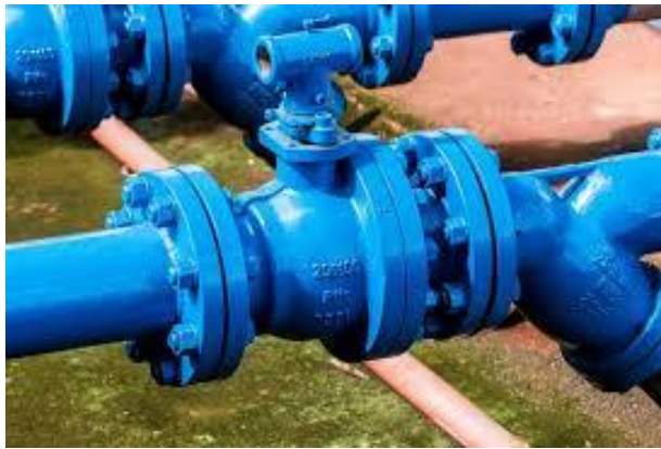
Gambar 1. 1 Instalasi ball valve 4100
